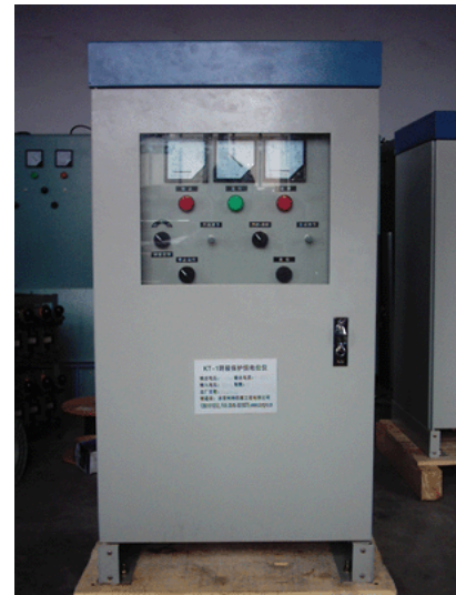
Air-cooled Transformer Rectifier
