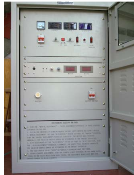
Operating module-type switching rectifier
